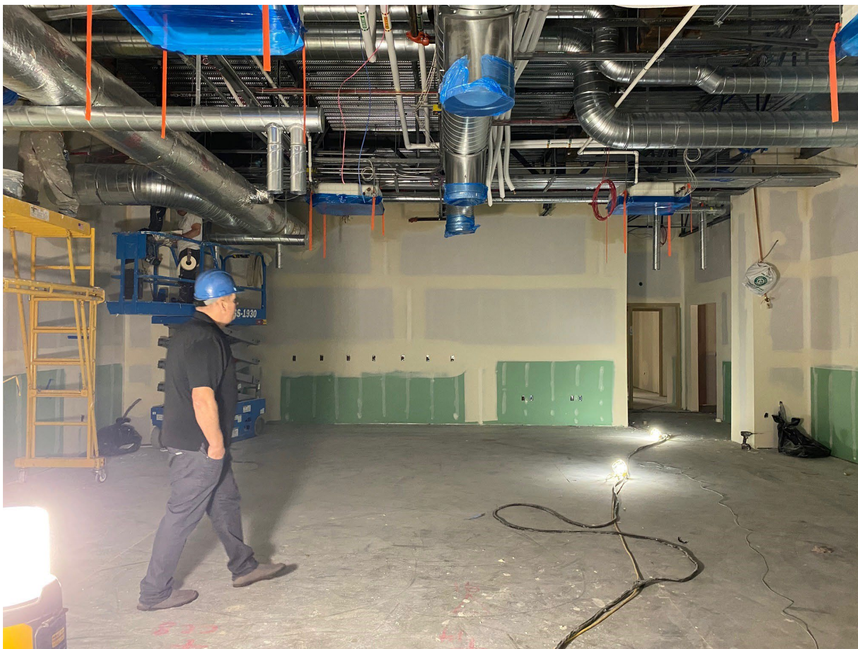
Federal Way Tox Lab – Instrument Room
