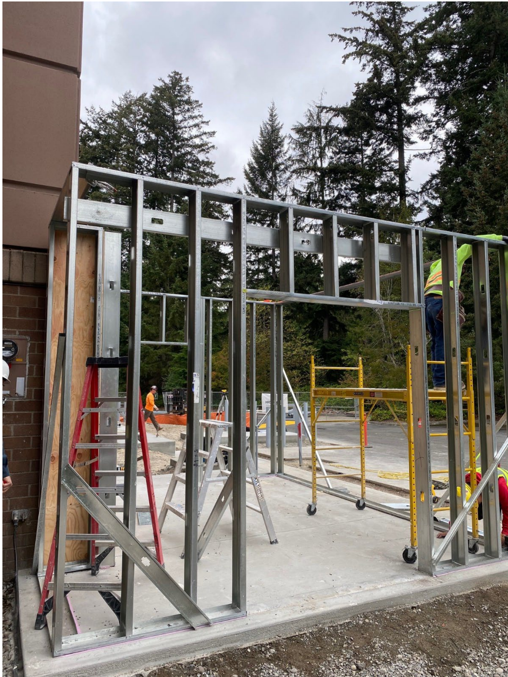
Federal Way Tox Lab – Conditioned Equipment Shed (N2)
